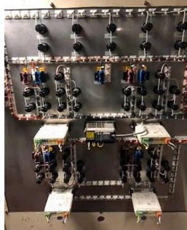
Relay Control System
